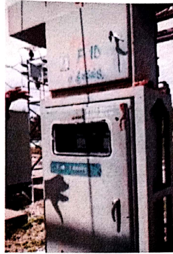
Figure 3.16: outside view of feeder
