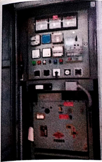
Figure 3.15: Inside view of feeder
