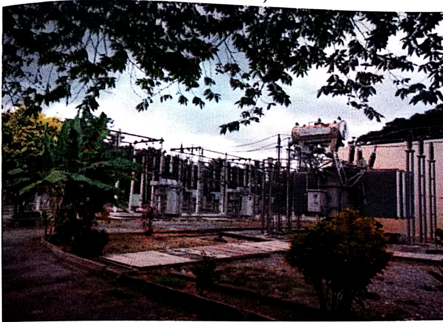
Figure 3.2: SUBSTATION VIEW OF SANTHEMAVATHURU
