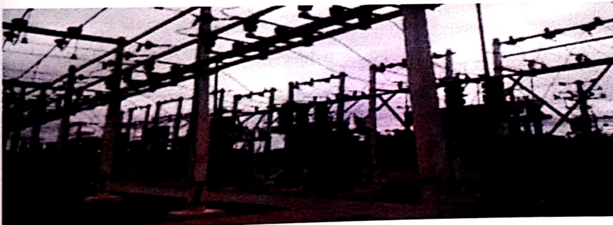
Figure 3.1(4b) OUT DOOR TYPE SUBSTATION
