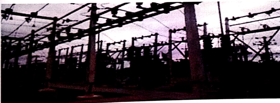
Figure 3.1(4b) OUT DOOR TYPE SUBSTATION
