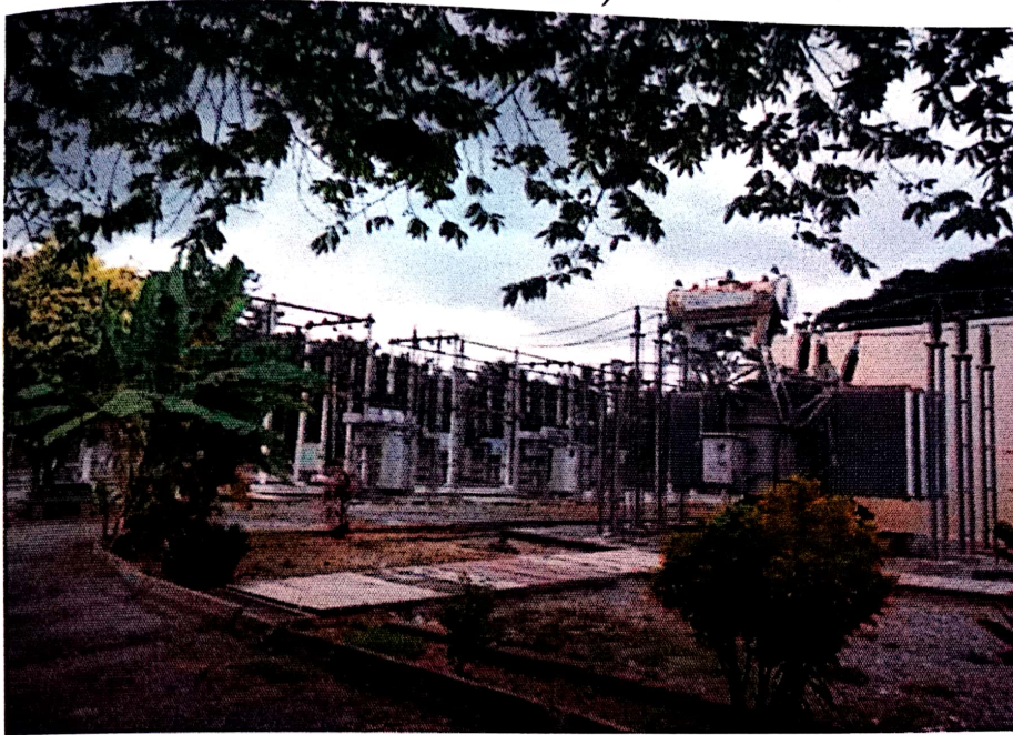
Figure 3.2: SUBSTATION VIEW OF SANTHEMAVATHURU
