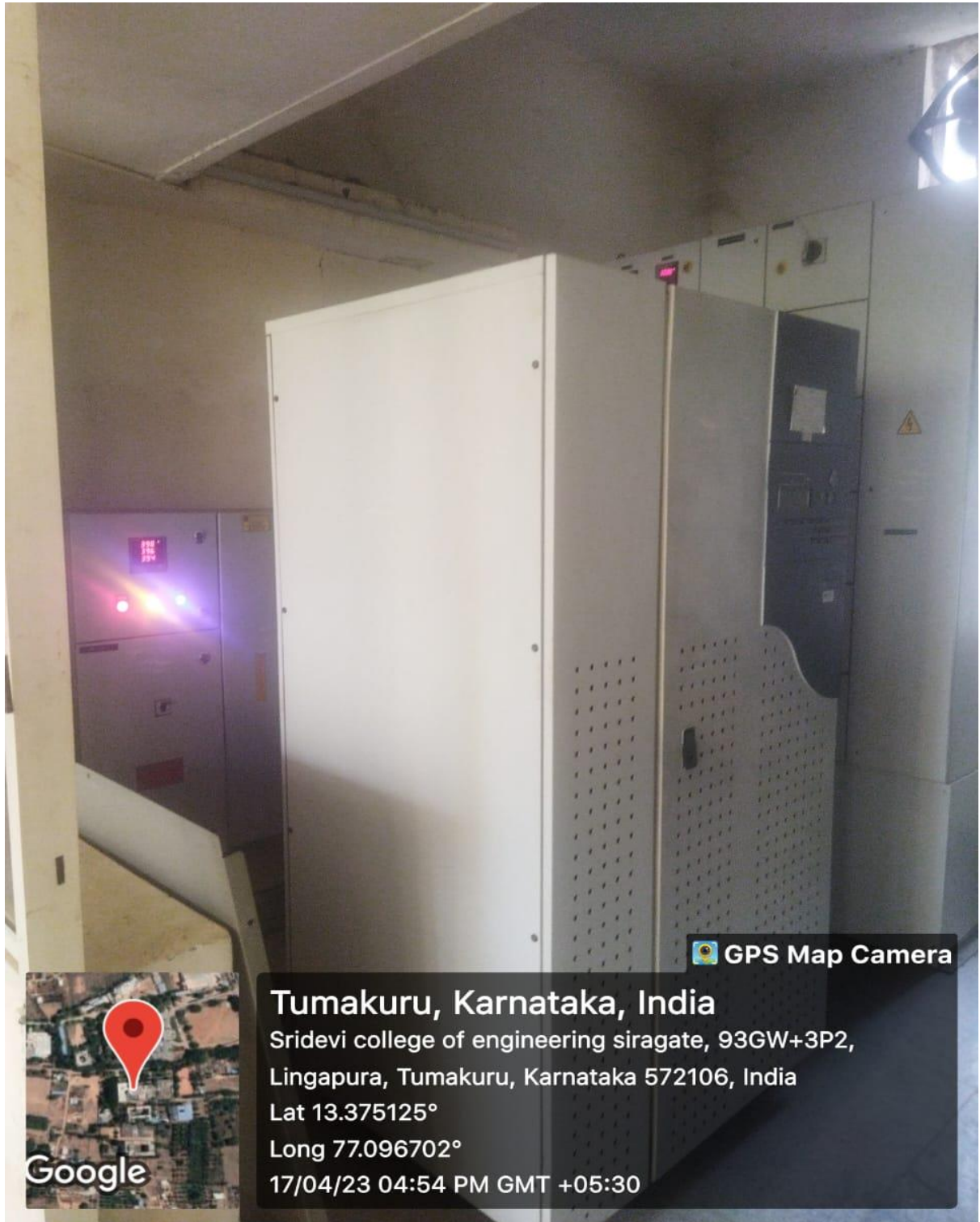
100 KVA Inverter Room
