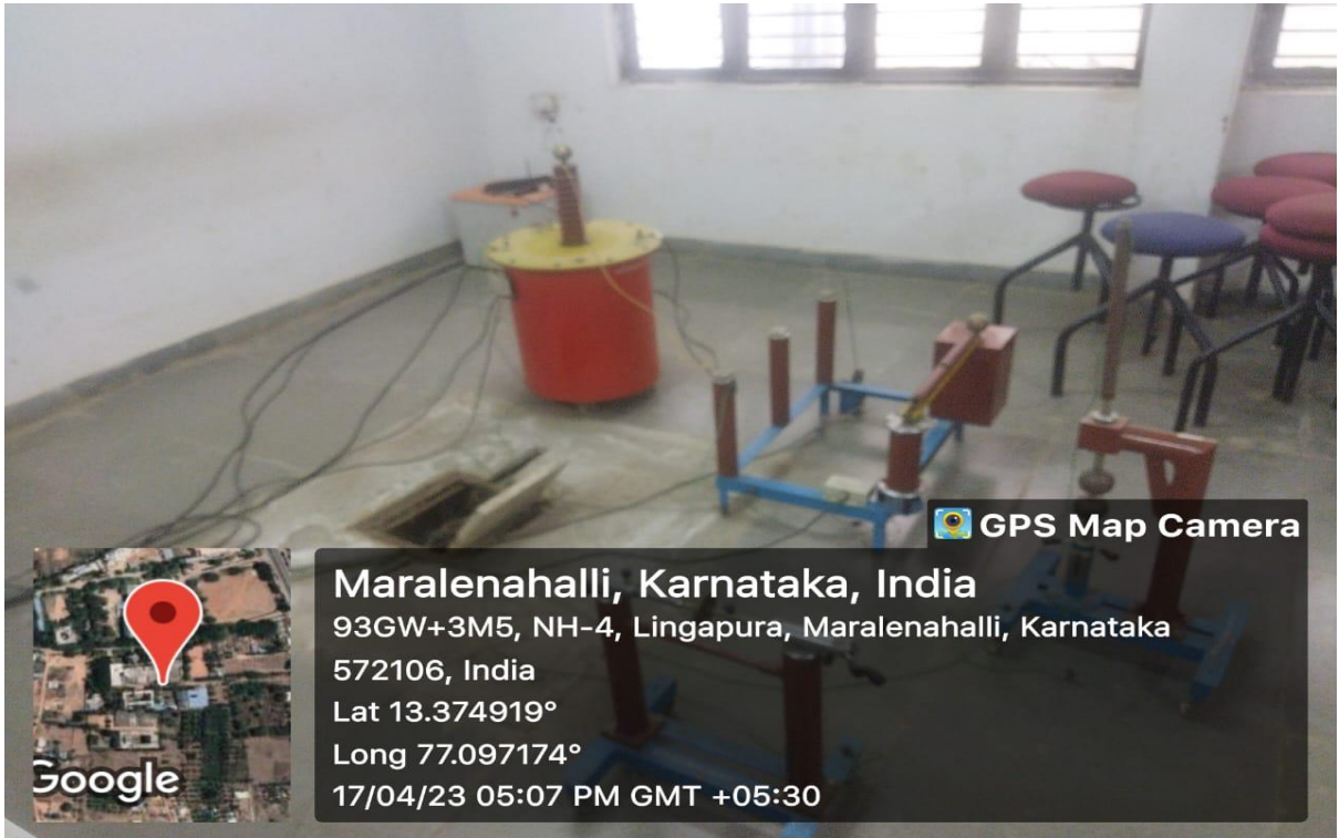
Electrical Engineering Department-Relay H V Laboratory
