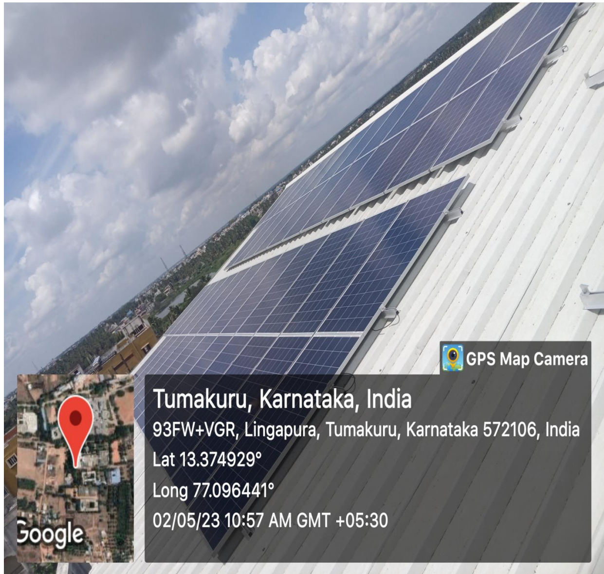
Solar Panel on the top of Auditorium
