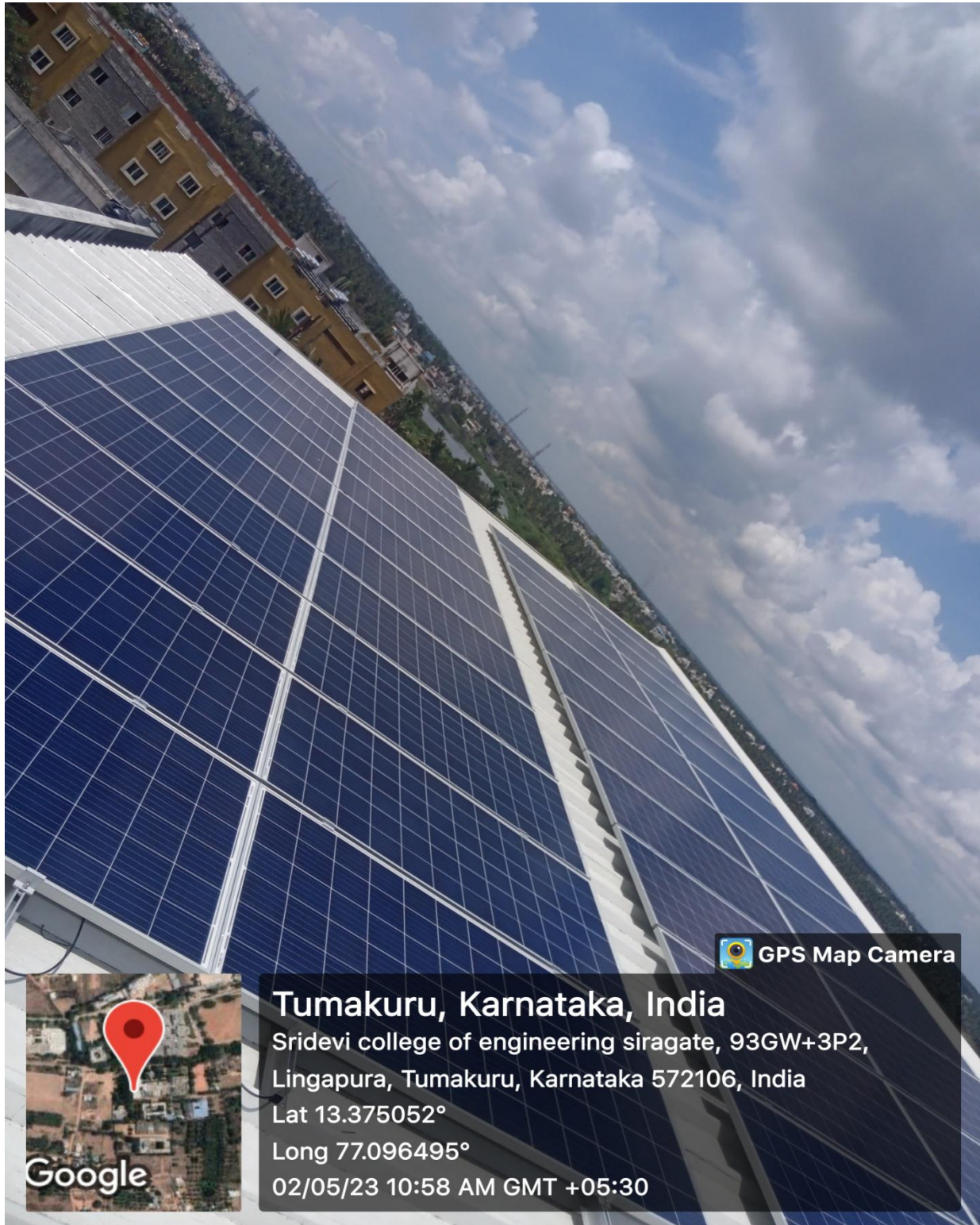
Solar Panel on the top of Auditorium
