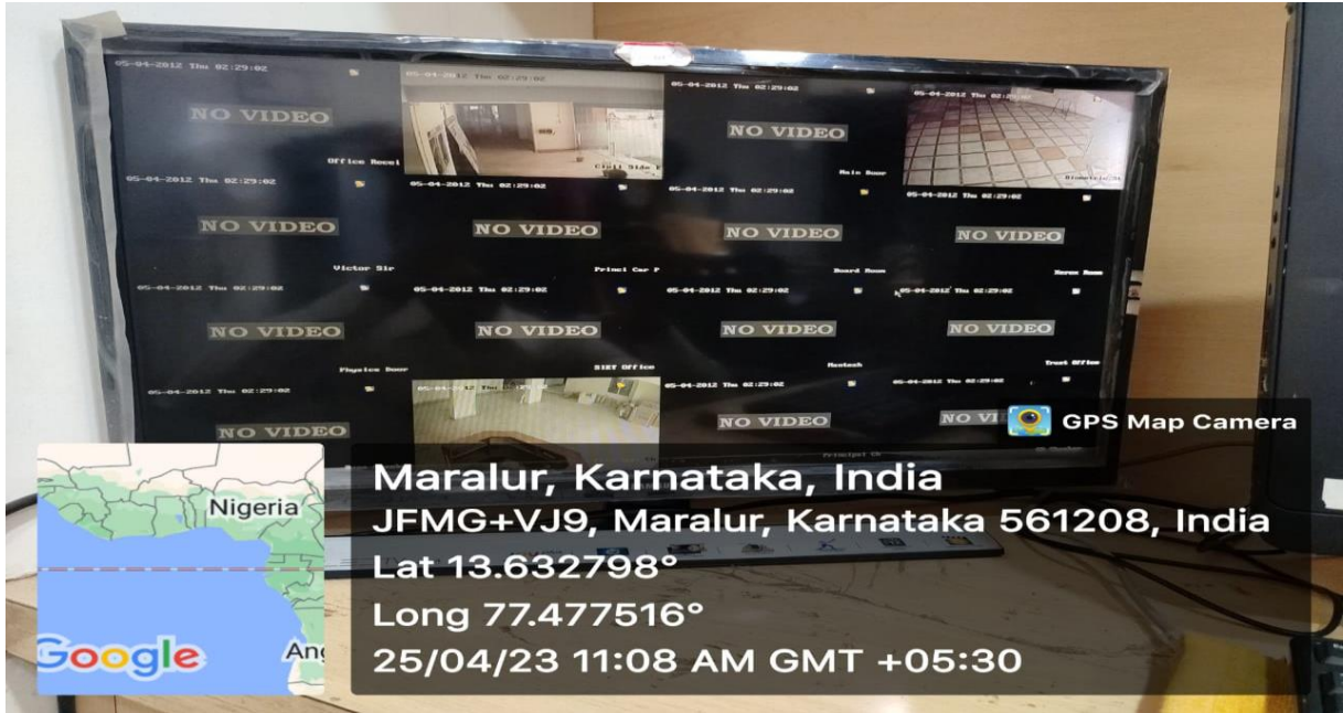
CCTV Monitoring and Footage at Trustee's Chamber
