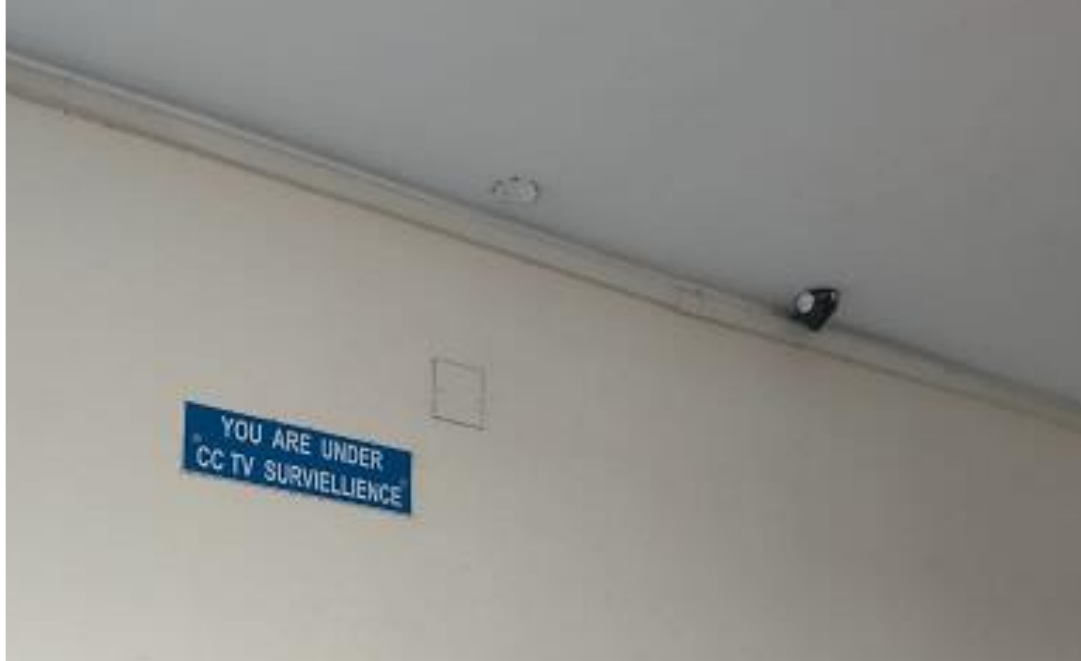
CC Camera installed in the SIET
