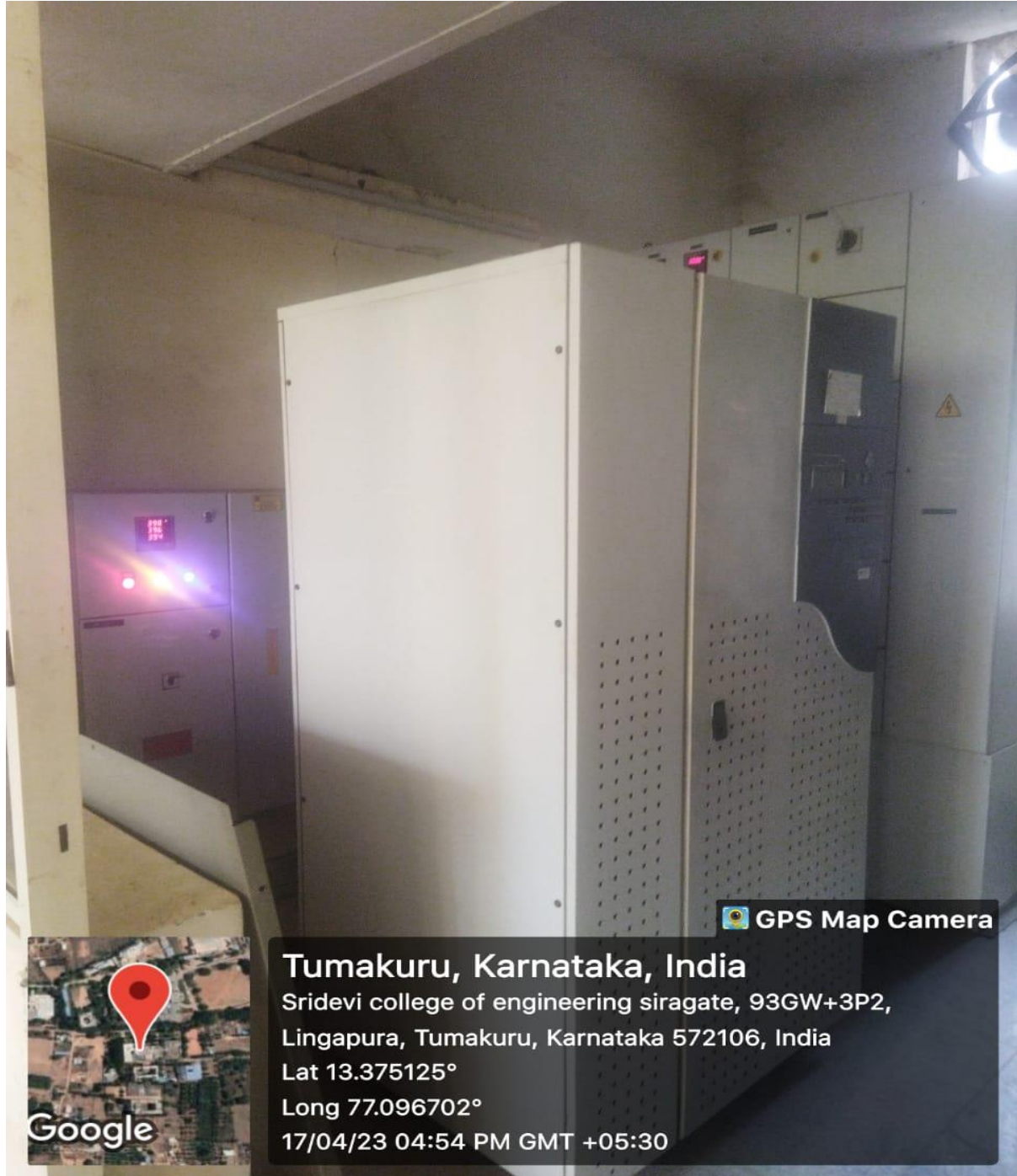
100 KVA Inverter Room
